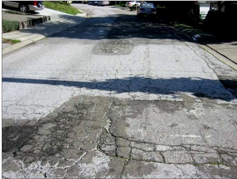
Figure 3.7 PCI <10 (Failed Condition)
