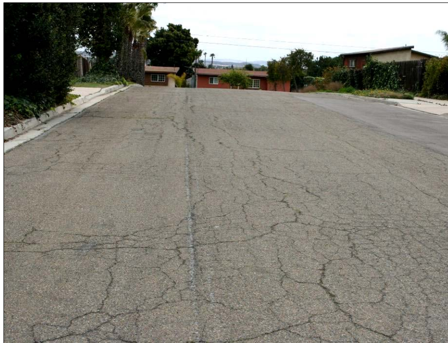
Figure 3.6 PCI = 40 (Poor Condition)
